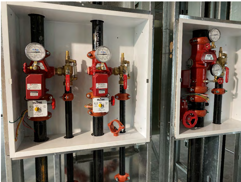
Sprinkler System - Level 2
