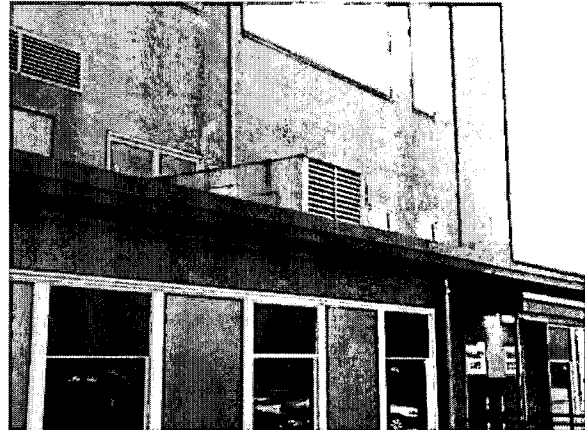
Cafeteria packaged rooftop unit
