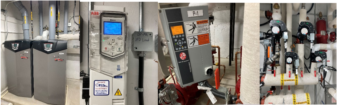
Figure 2 – Skwo:wech Elementary energy efficient heating system.
